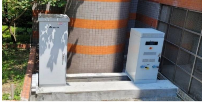
Figure 10. The 100 kW/50 kWh Energy Storage System in Baoshan Campus
