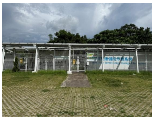
Figure 9. The 1 MW/1.26 MWh Energy Storage System in Baoshan Campus
