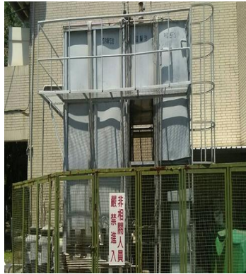
Figure 2. Jinde Campus Wastewater Treatment Plant
