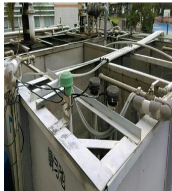
Figure 3. Jinde Campus Wastewater Treatment Plant
