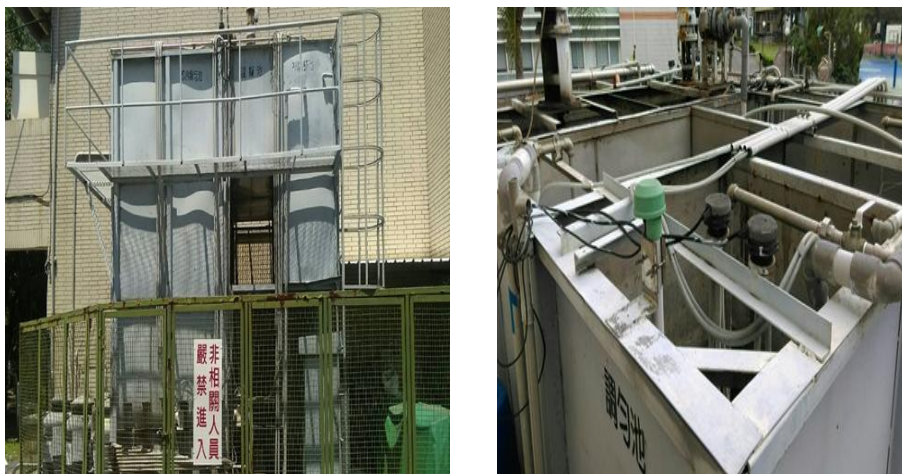
Figure 2-3. Jinde Campus Wastewater Treatment Plant
