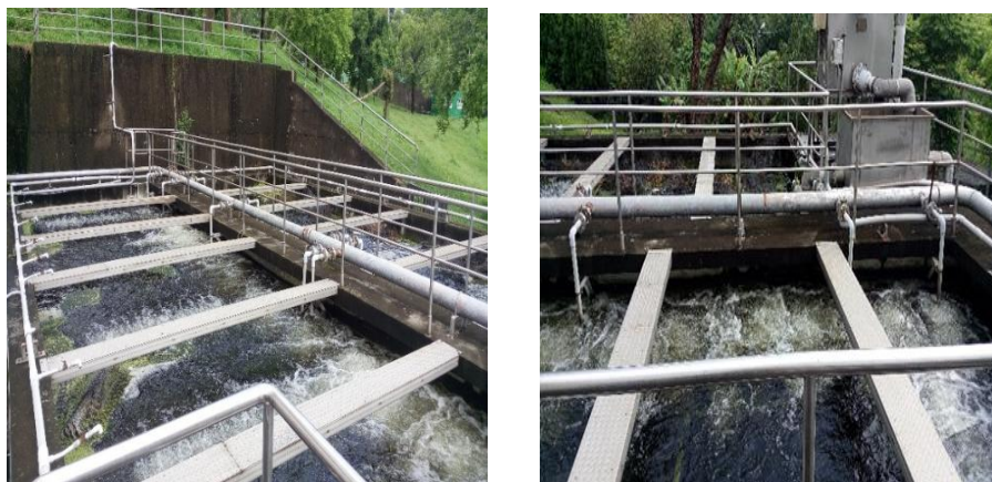
Figure 4-5. Baoshan Campus Wastewater Treatment Plant
