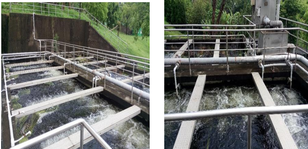
Figure 4-5. Baoshan Campus Wastewater Treatment Plant
