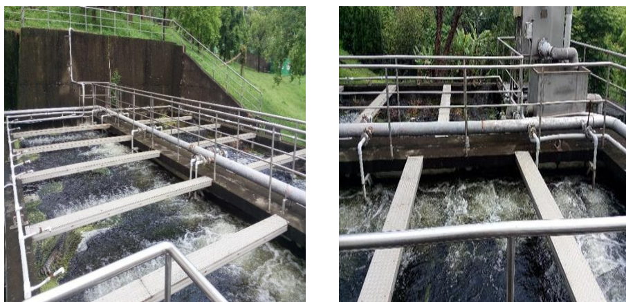
Figure 4-5. Baoshan Campus Wastewater Treatment Plant
