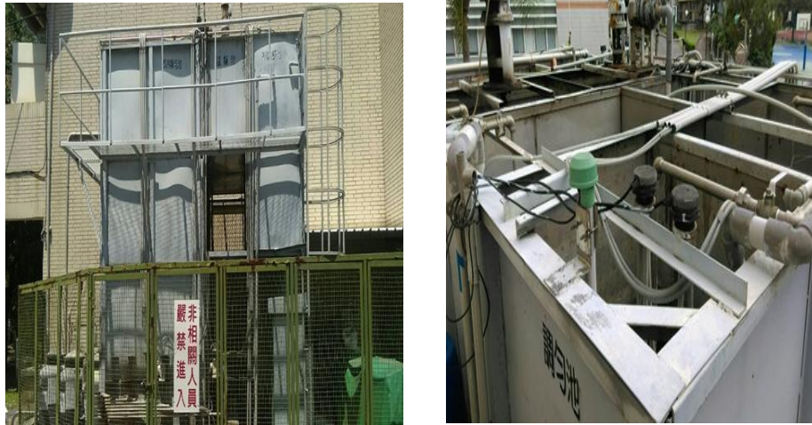
Figure 2-3. Jinde Campus Wastewater Treatment Plant
