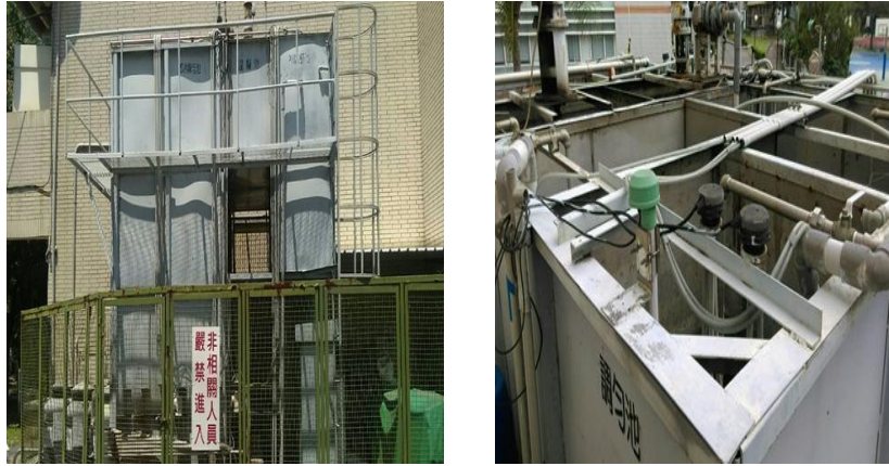
Figure 2-3. Jinde Campus Wastewater Treatment Plant
