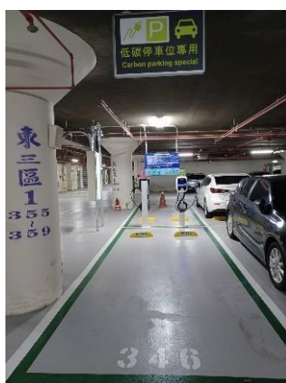
Figure 8. Electrical Car Charging Station at NCUE's Jinde Campus Parking Spaces
