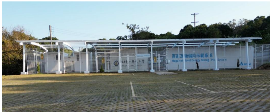
Figure 3. Megawatt-Scale Energy Storage System
