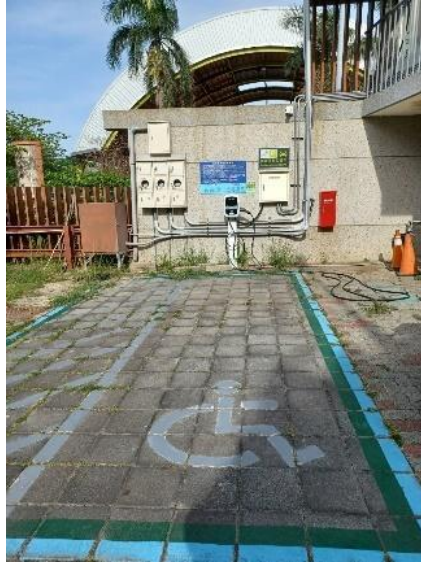
Figure 5. Charging Station at NCUE Baoshan Campus Parking Spaces
