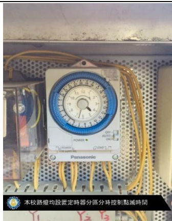
Figure 11: All street lights on campus are equipped with timers for zoned and time-controlled activation
