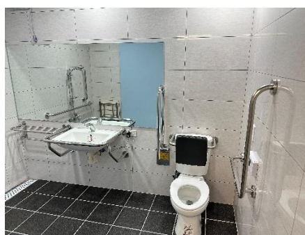
Figure 16: Accessible facilities in dormitory toilets
