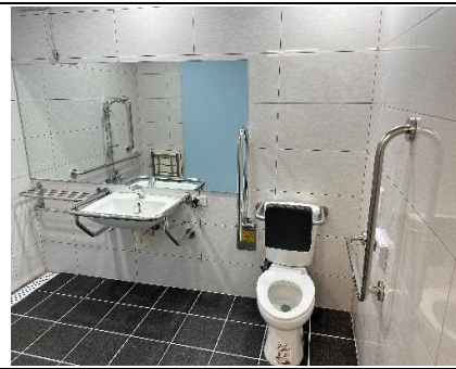
Figure 10: Accessible facilities in dormitory toilets
