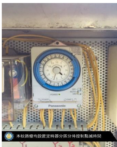
Figure 13: All street lights on campus are equipped with timers for zoned and time-controlled activation
