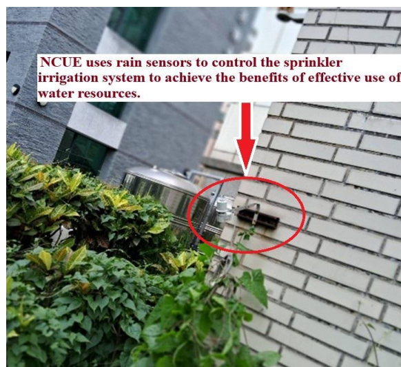
Figure 3: The above picture shows that NCUE uses rain sensors to control the sprinkler irrigation system to achieve the benefits of effective use of water resources.
