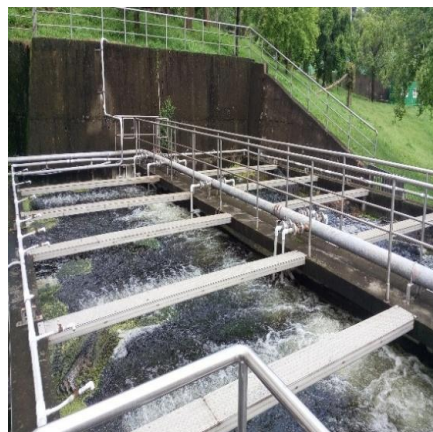
Figure 4. Sewage Treatment Plant on Baoshan Campus
