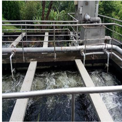
Figure 5. Sewage Treatment Plant on Baoshan Campus
