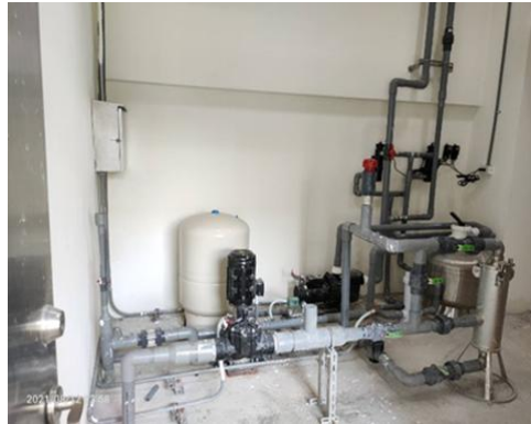
Figure 3. Irrigation system at 10th Dormitory at the Baoshan Campus
