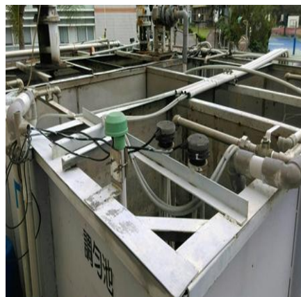
Figure 3. Sewage Treatment Plant on Jinde Campus
