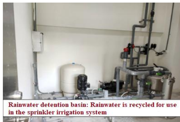
Figure 4: Rainwater detention basin: Rainwater is recycled for use in the sprinkler irrigation system
