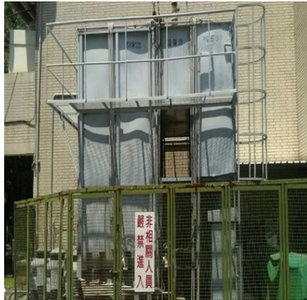
Figure 2. Sewage Treatment Plant on Jinde Campus
